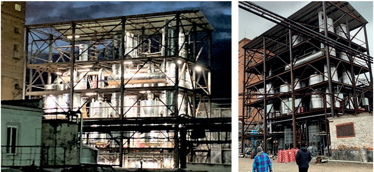
Fig. 5. External view of the evaporation plant
