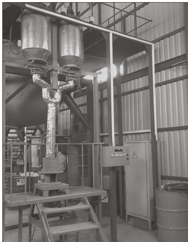
Fig. 6. The plant for preparing BLE
