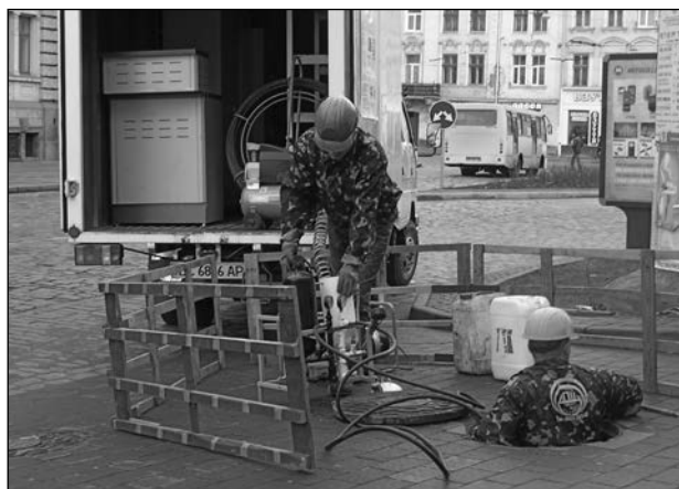
Fig. 3. Mobile diagnostic and recovery complex during repair of sewer collector on Svobody Avenue in Lviv
