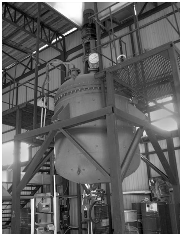
Fig. 5. The reactor of pilot plant for production of «A» polyol components of polyurethane injectable materials
