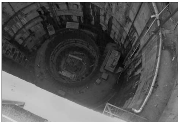
Fig. 10. The reinforced concrete pit of turbine room at the Dniester HEPS repaired using injectable composites to prevent water infiltration
