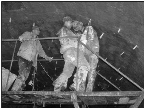
Fig. 2. Techno-Resource workers drilling holes for injection into a sewage collector on Svobody Avenue in Lviv
