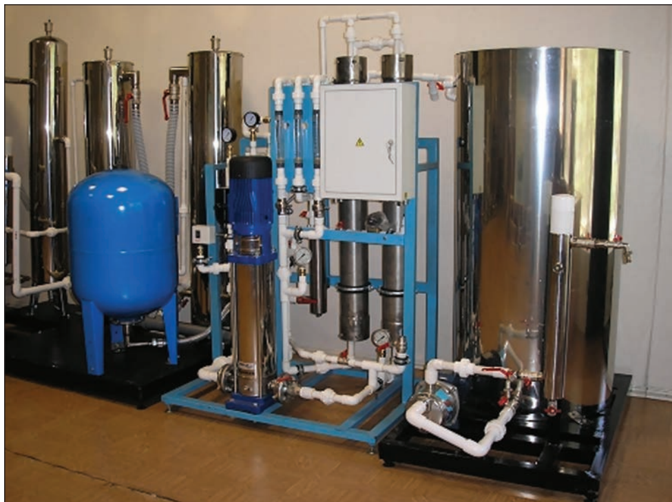
Fig. 2. Stand-alone installation for collective use, capacity of 0.5 m 3 /h
