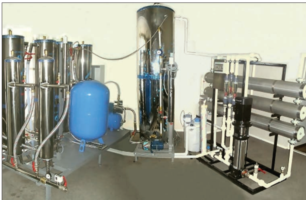
Fig. 1. Stand-alone installation for collective use, capacity of 5 m 3 /h
