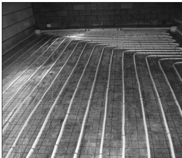
Fig. 16. Heat exchanger (floor water circuit heating system)
