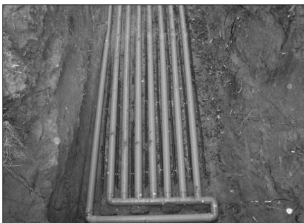
Fig. 14. Ground–air heat exchanger
