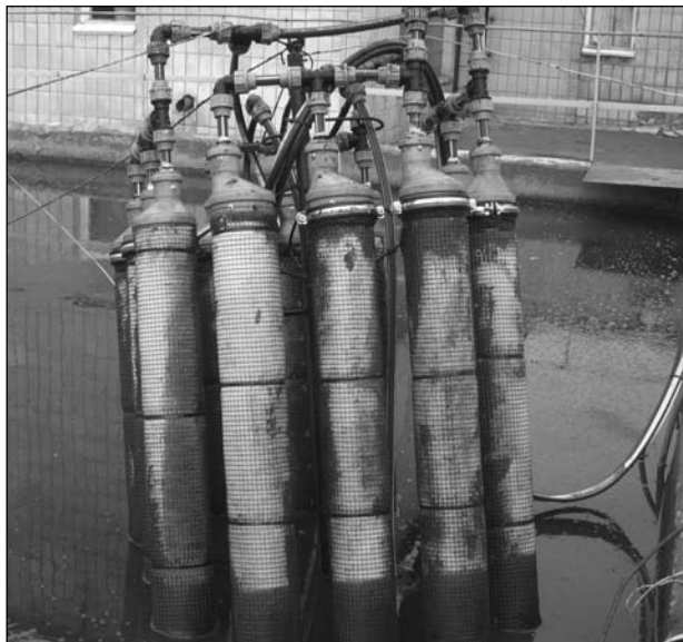
Fig. 7. The filter module after regeneration
