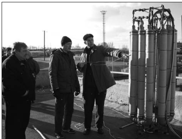
Fig. 2. Picture of the pilot facility filter module
